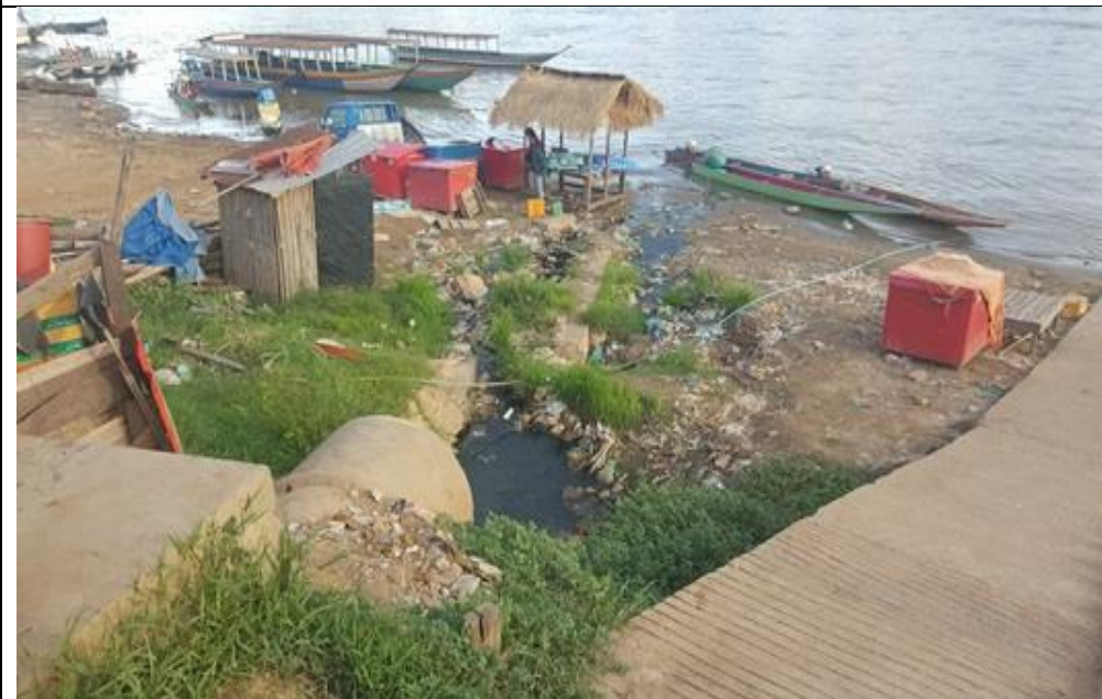
Figure 11b: Stormwater drainage pipe and outfall to Mekong to be relocated downriver
